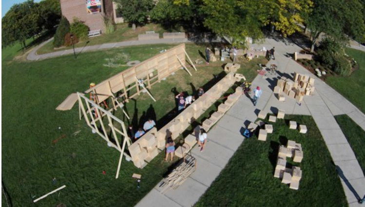
Figure 2: Sukkah construction underway on the University of Hartford campus; elements prefabricated by students are assembled and will be disassembled after the festival of Sukkot. Photo: Rebecca Tuscano-Moss
