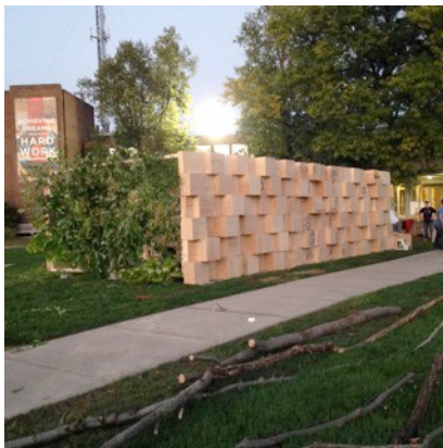
Figure 3: Natural, unprocessed materials such as saplings and phragmite are set in place in the sukkah's end wall. Photo: Rebecca Tuscano-Moss
