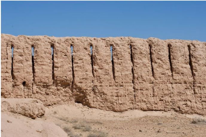
Figure 4: Eroding walls of Ayaz Qala, Karakalpakistan returning to the earth from which they were constructed. (Ray Stevens).
